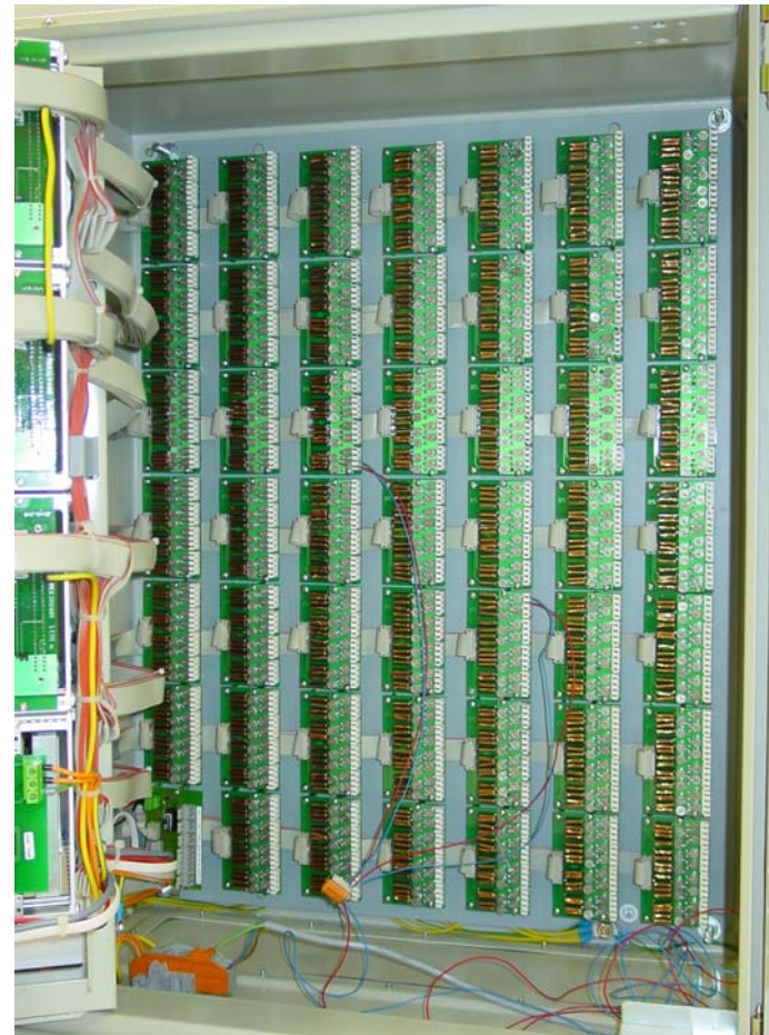
LCU (inside cabinet)
